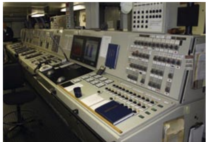
ABOVE: A typical air-conditioned engine control room from where a ship's main engines, generators and on board systems are monitored and controlled.
